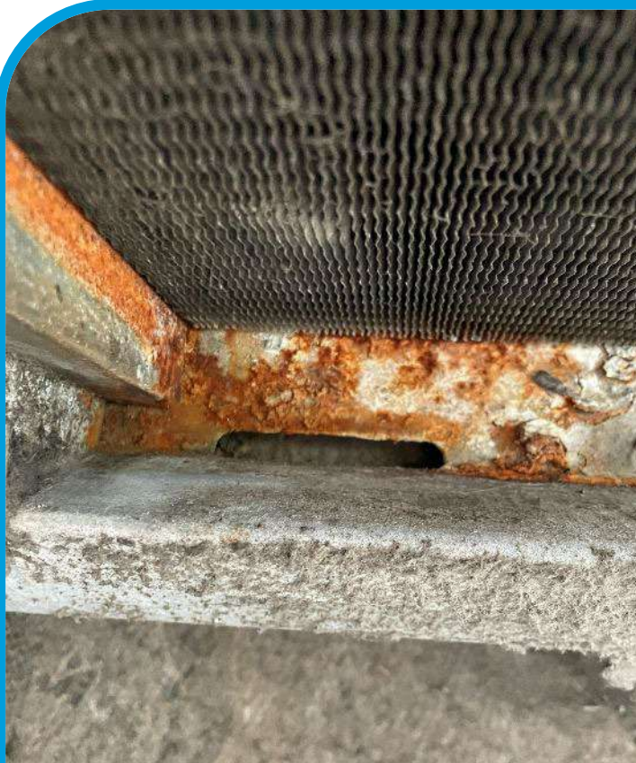
Rust and debris in pan
