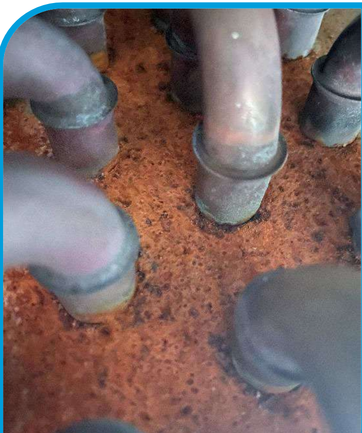
Rust and debris
