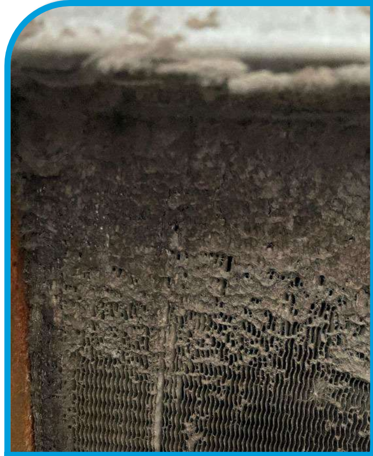
Top of clogged coil
