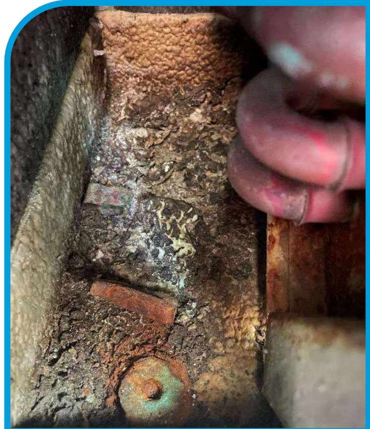
Rust and debris in pan
