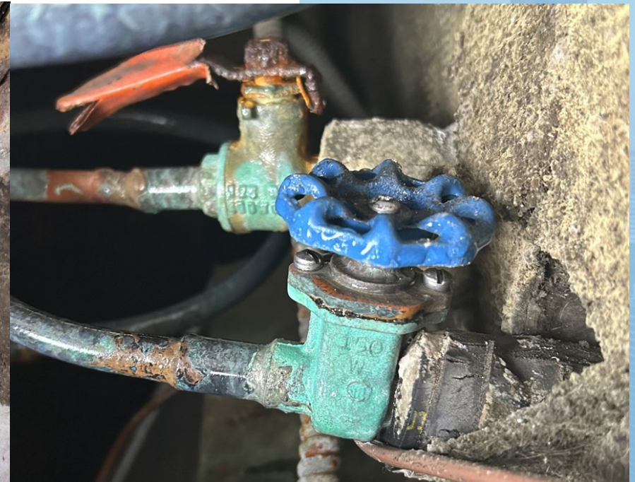
Valves should function in the event of a service emergency.
