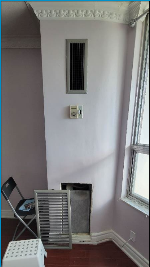
1. Unable to Access FCU through narrow opening
