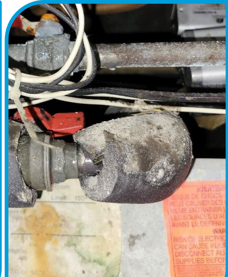
On Pipe Insulation
