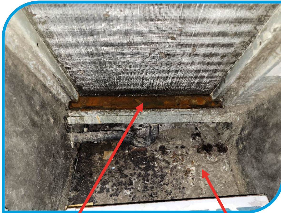
Water overflowing from pan
