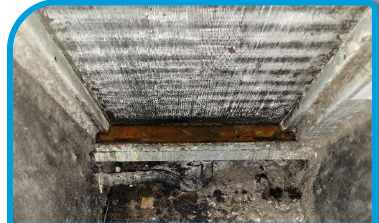
Drain pan compromised + Leak
