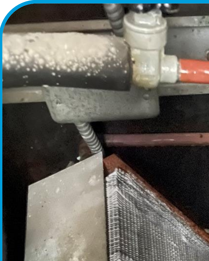
On hose insulation
