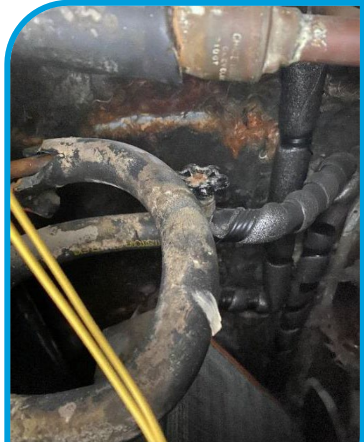
On Insulation throughout
