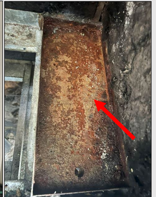
Scale Erosion on Drain Pan, no flood sensor
