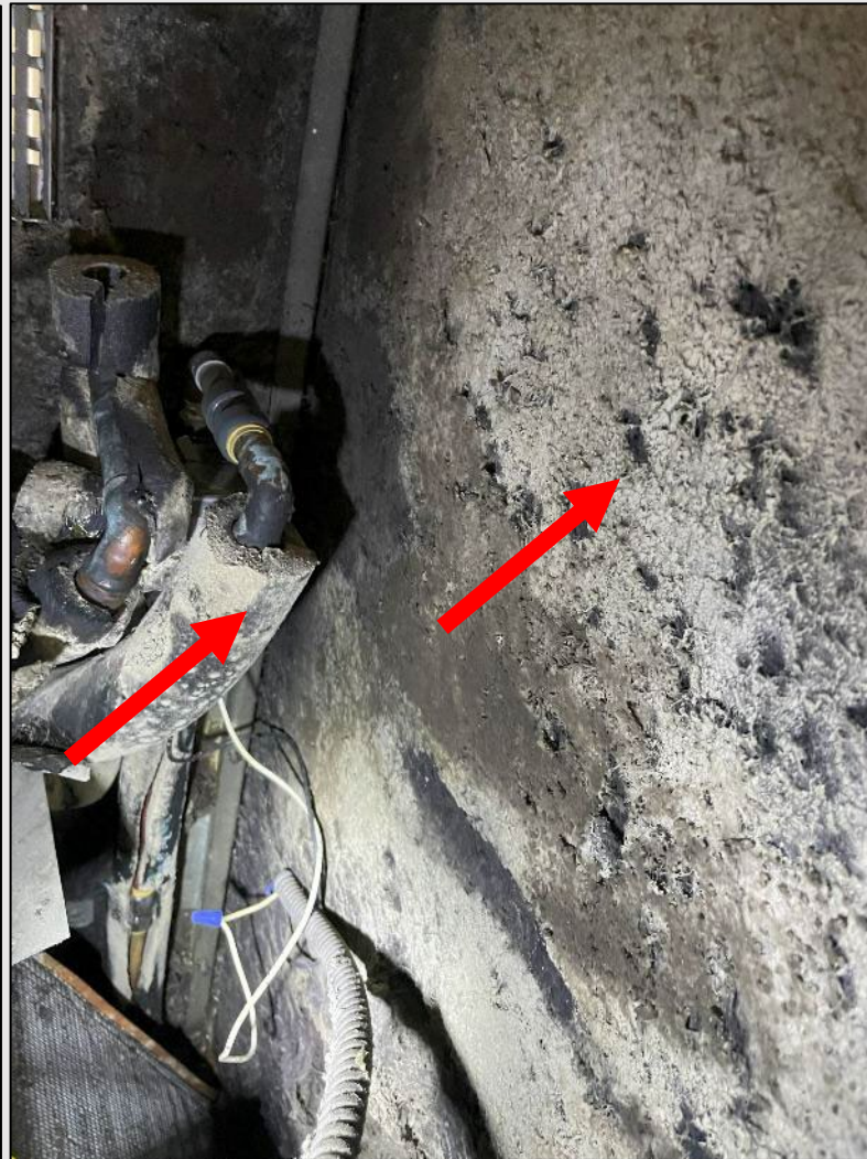
Side Wall of Cabinet and Pipe Insulation
